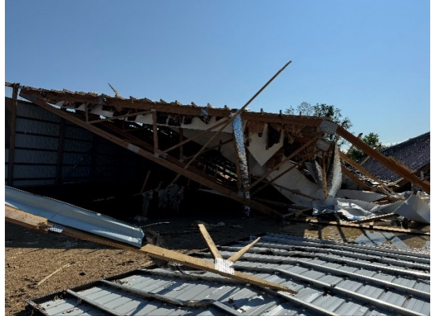
A collapsed horse arena on Brundige Rd., Elburn.
